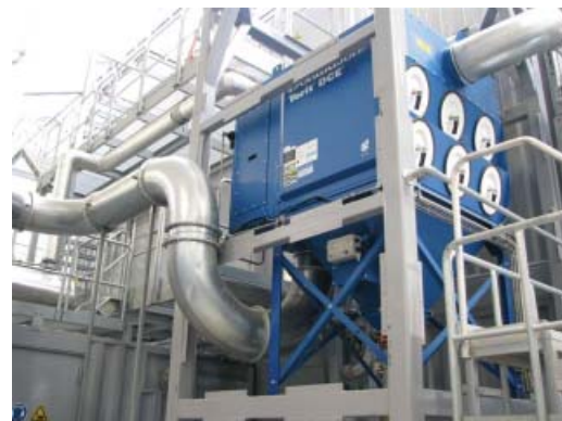
Static Detonation Chamber 1200 used at Anniston's Chemical Agent Disposal Facility
